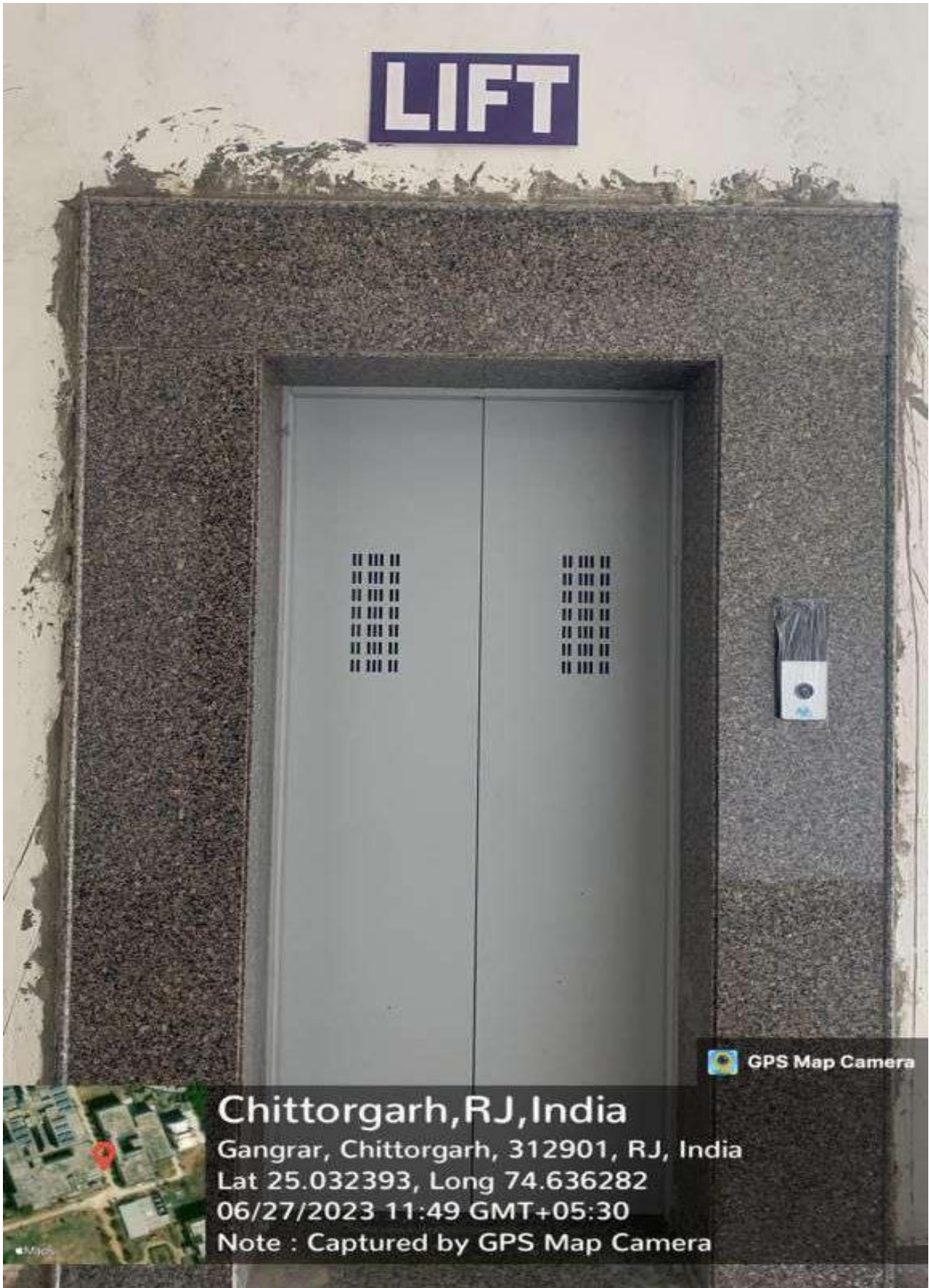
Lift facility (Engineering Block)
